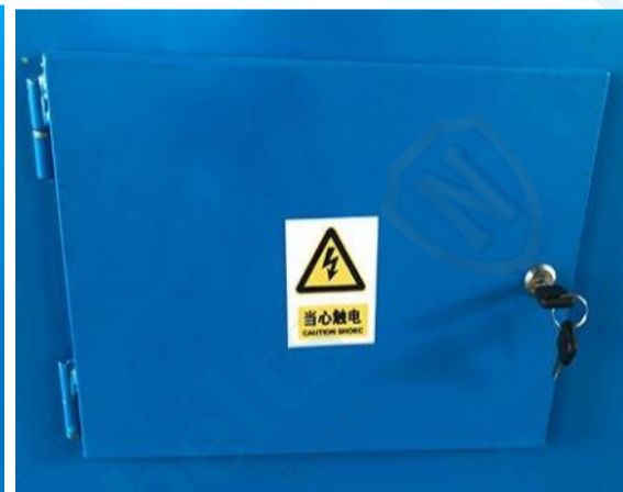
Control panel with cover door to protect the buttons
