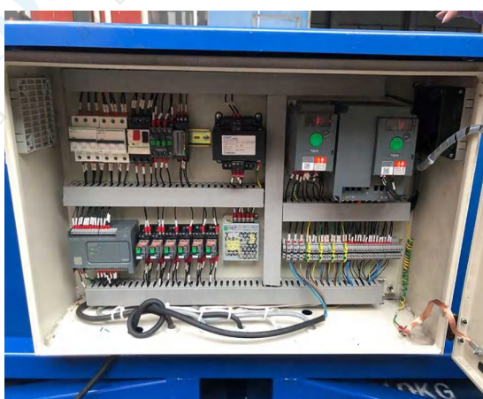
Main control box with Schneider VFD
