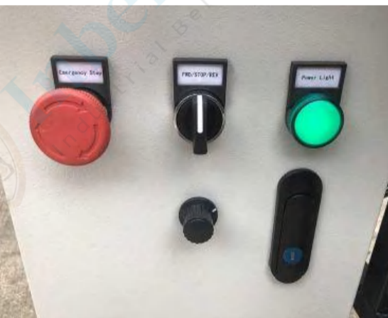
Control Panel for Conveyor Operation
