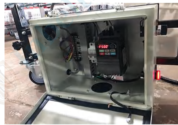
The control box with inverter to adjust speed.
